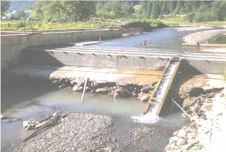
Water intake structure with “fish ladder” of the Probiynivs'ka SHPP-2 (232 kW) (photo by O. Vasyliuk)
